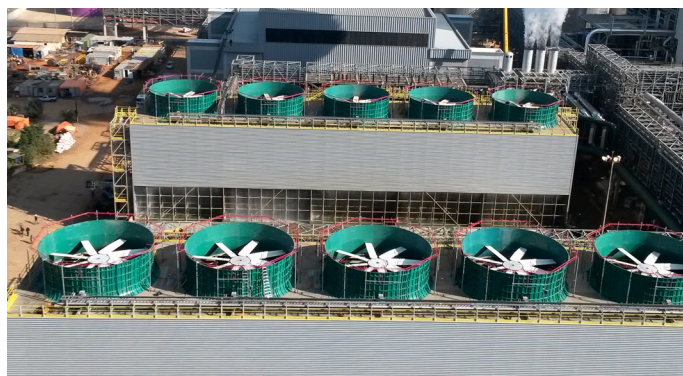
Induced Draft Counterflow CT in Brasil
