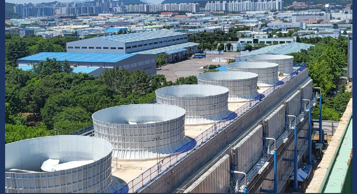
Hybrid Cooling Tower in South Korea
