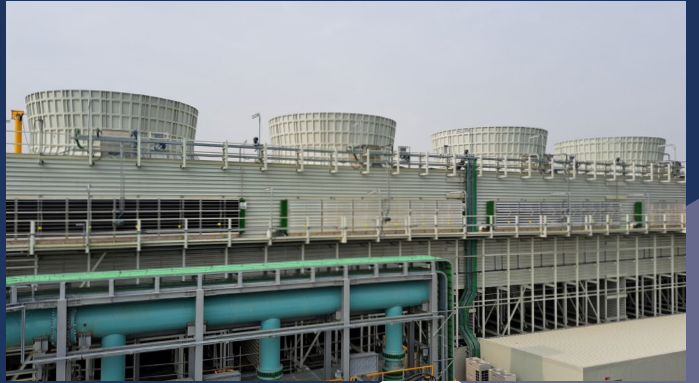
Hybrid Cooling Tower in Italy
