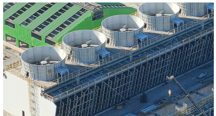
Crossflow Cooling Tower in Algeria
