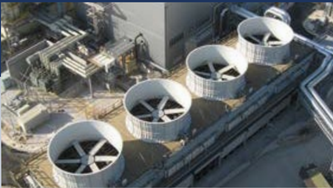
Hybrid Cooling Tower in South Korea
