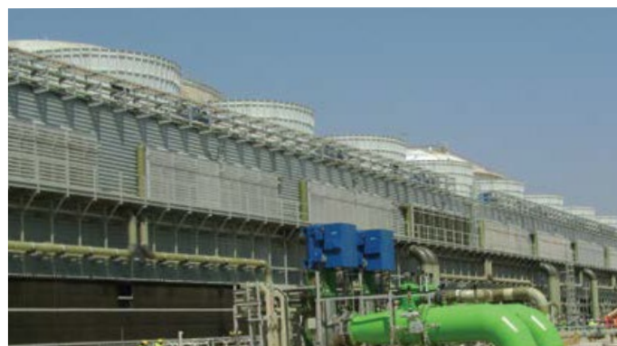
Seawater Cooling Tower in Spain
