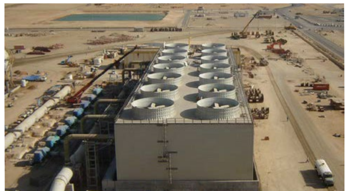
FRP Cooling Tower in Saudi Arabia
