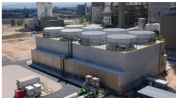
Noise-abated Cooling Tower in Portugal
