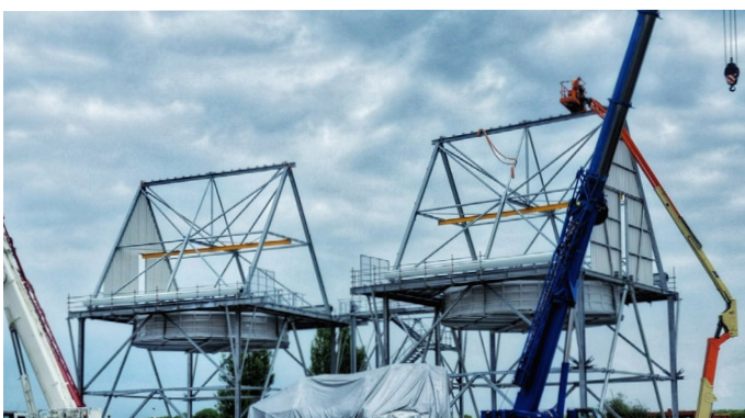
Air-Cooled Condenser installation in UK
