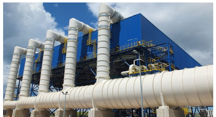
Air Cooled Condenser in Turkey
