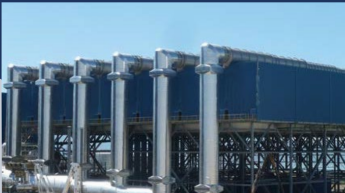
Air-Cooled Condenser in Turkey
