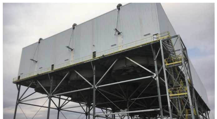
Air-Cooled Condenser in South Africa
