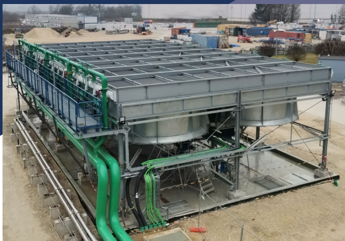
Air Fin Cooler in Germany
