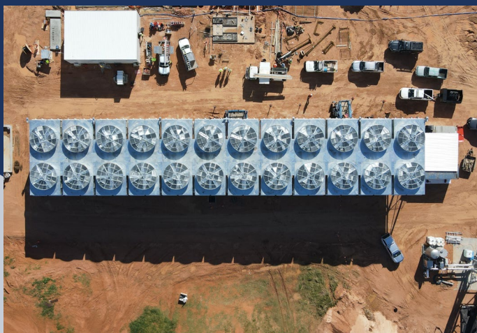
Air Fin Cooler in Australia
