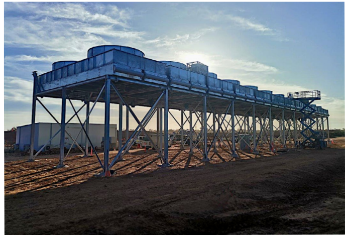
Air Fin Cooler in Australia
