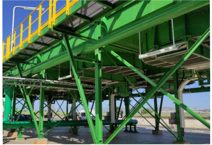
Air Fin Cooler in Spain
