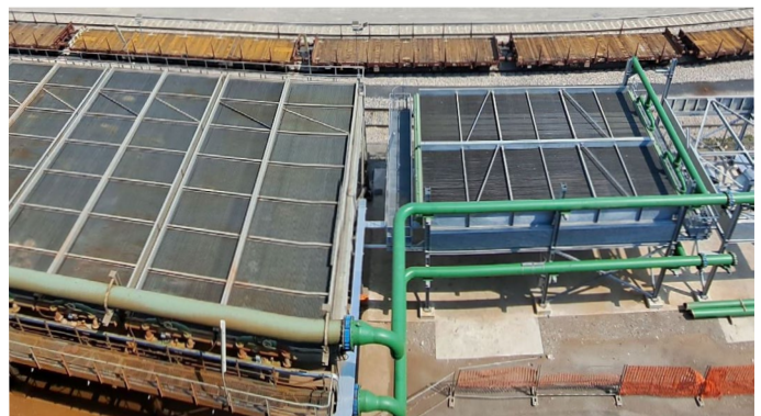
Air Fin Cooler in Italy
